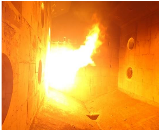
Boiler first fire
